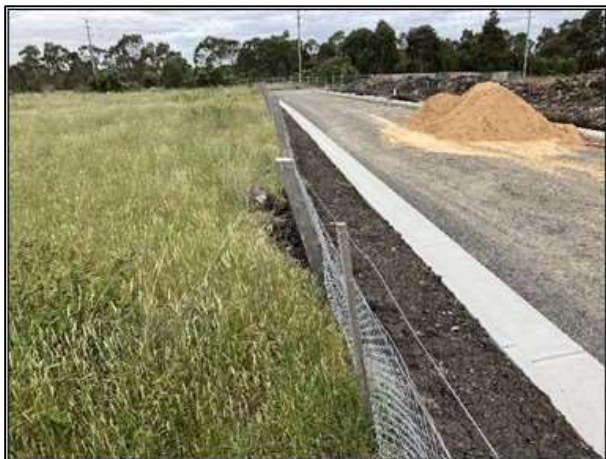
Plate 43. Implemented kerb leveling out soil within offset site and adjacent construction zone (Ecology and Heritage Partners Pty Ltd 01/11/2023).
