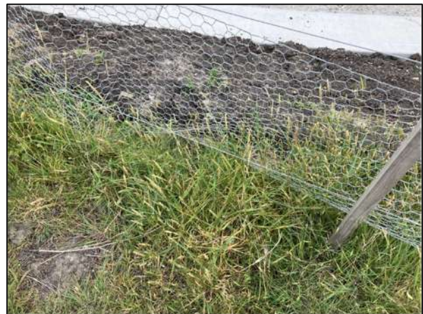
Plate 44. Rabbit proofing lifting along eastern fence, adjoining construction works (Ecology and Heritage Partners Pty Ltd 01/11/2023).
