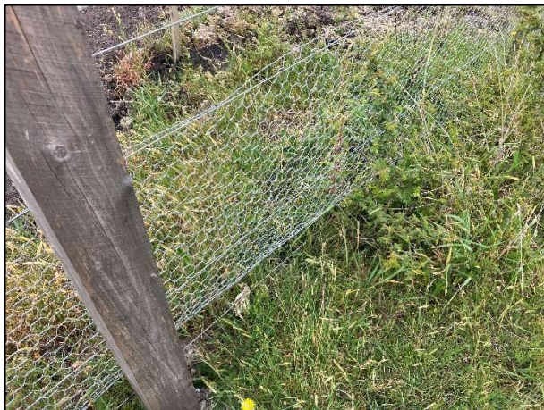
Plate 31. Gap underneath eastern fence rabbit proofing (Ecology and Heritage Partners Pty Ltd 01/11/2023).
