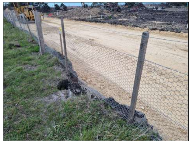
Plate 42. Interim soil barriers implemented to prevent further erosion (Ecology and Heritage Partners Pty Ltd 24/08/2023).
