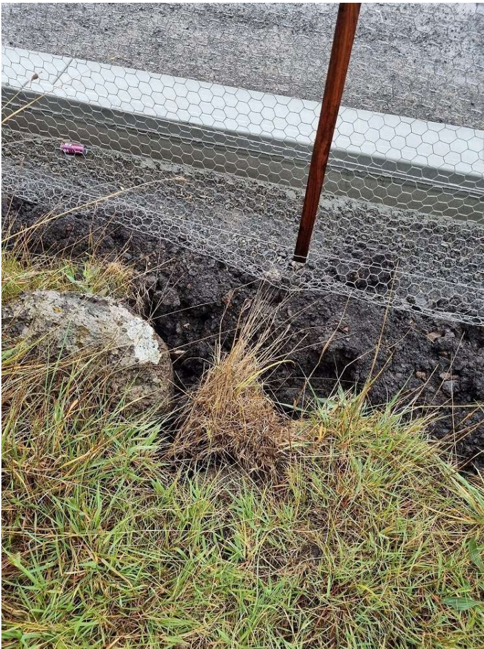
Area along eastern boundary that will require erosion repairs
